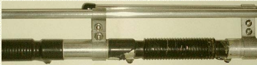
Water got inside a trap due to cracked heath shrink tubing.
